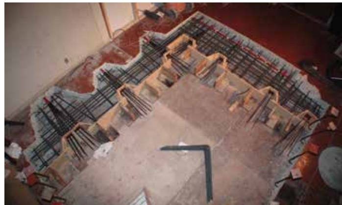
Figure 3. Slab opening with antiquated button-headed wire system.
